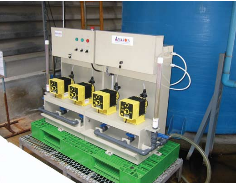
亚马逊化工参与项目的启动，这可以以确保定量给料设备尺寸的精确与完整性，及其能够与纸厂DCS连接 Amazon's participation in start-up projects ensures that the dosing equipment is correctly sized, integrated and linked to the mill's DCS
