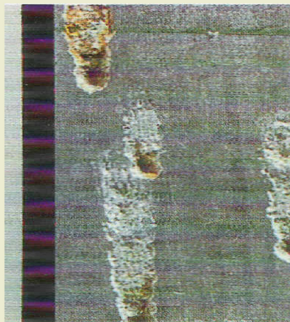
Figure 4. Pitting corrosion caused by microbiological attack
